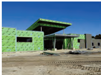
The new Howard T. Ennis School is being constructed on a parcel of land on Patriots Way north of Millsboro across from Sussex Central High School.
